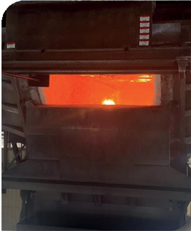
Aluminium Remelt Furnace.
